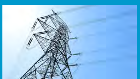
High-voltage substation – energy Zeebrugge partnership – ELIA
